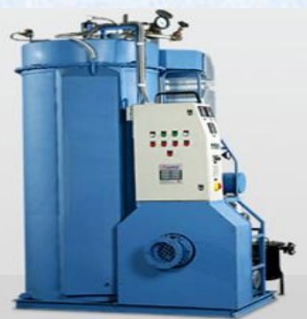
Existing boiler Diesel fired
